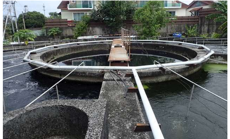
円形のSTP (5,000PE)
