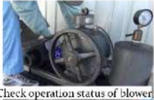
Check operation status of blower
