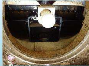
Outlet of treated water of Johkasou
