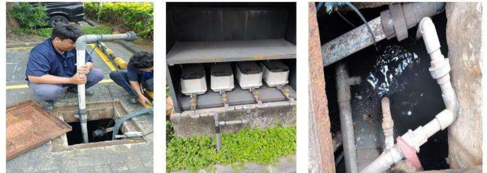
Case F Hotel : Restoration Project, installation 4 unit YASUNAGA LW 240
