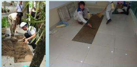
the soil and decorative tiles on top of the manhole had to be removed before the maintenance work
