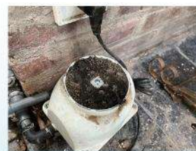
Clogging of air filter (Example)
