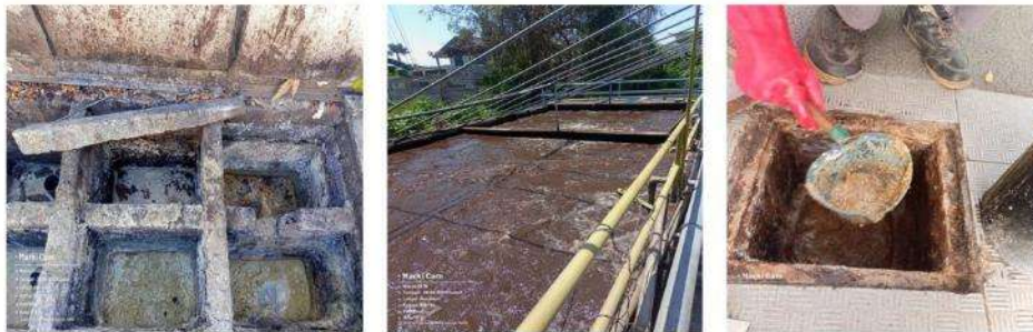
Case E Hotel : 1. Outdated wastewater treatment facility 2. Improper design
