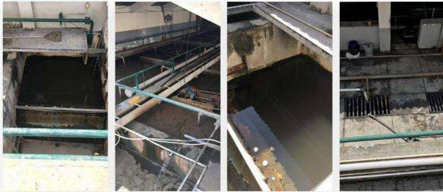
Case Hotel C : Sludge Carry over due to improper Operational & Maintenance
