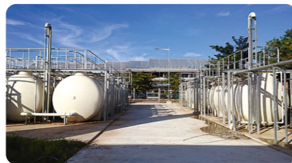
Vientiane Airport terminal (Laos: 250 m 3 /day) Source: Kubota Johkasou System Co.,Ltd
