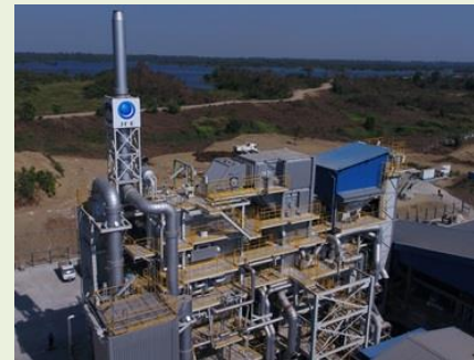
Incineration plant (60t/ day) completed in April 2017 in Yangon
