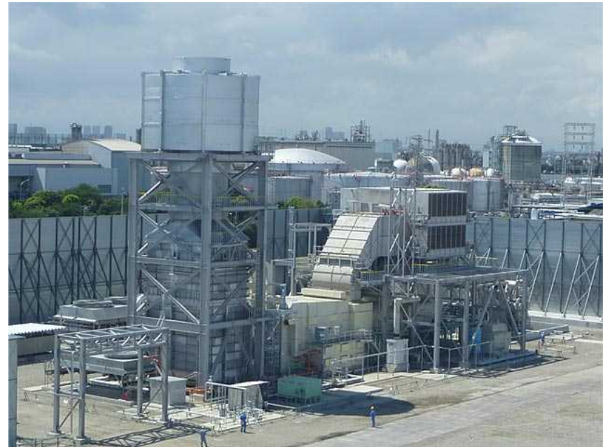
SPGF installed at Kawasaki Thermal Power Plant *2
