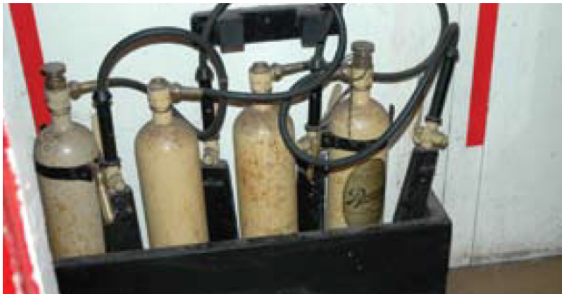
One of several sets of original fire extinguishers
