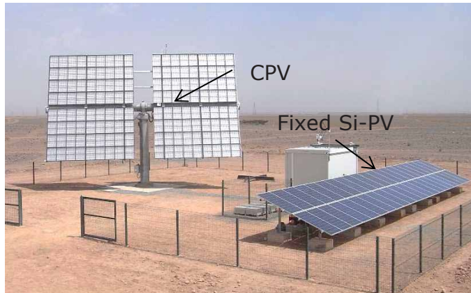
CPV in Ouarzazate (2015-2016)
