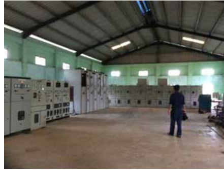
Electric Room (PV –related Equipment can be stored)
