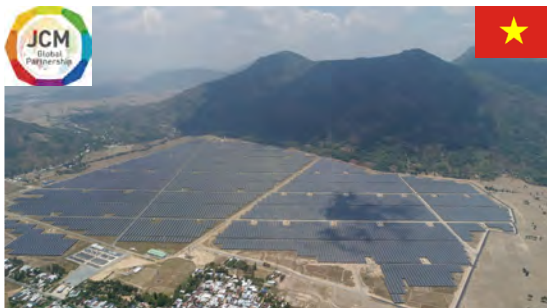
106MW Solar Project in An Giang Province, Vietnam
