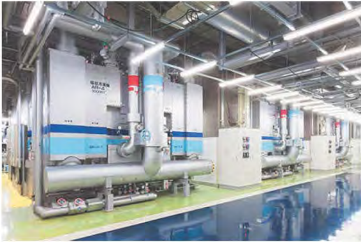
District heat plant supplying to Minato Mirai 21 One of the world's largest inverter-driven turbo chillers
