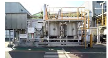
CFC Recovery EQP.
