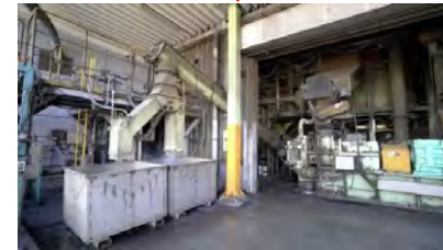
Heating CFC Separator
