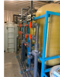
Seawater Desalination Equipment (Peleliu)
