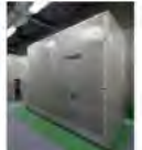
NaS battery in Miyako-Island
