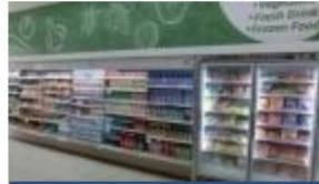
Energy saving at convenience stores, Panasonic, Indonesia
