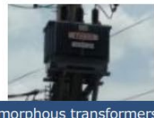
Amorphous transformers in power distribution, Hitachi Materials, Vietnam
