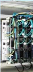
• Wired Telecommunications Equipment Construction
