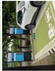
7kW & 22kW EV Charging Stations (59 vehicles charged since March 2024)
