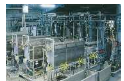
Fluorocarbon destruction facility
