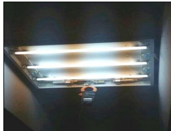
Stairways (fluorescent Lamps)
