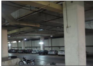
Loading Bay & Service Tunnel (fluorescent Lamps)
