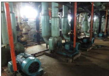
Chilled Water Pumps
