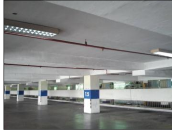
Parking (fluorescent Lamps)
