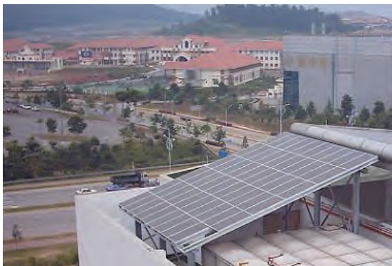
PV Panels on the roof top
