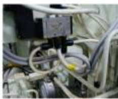
point: hose joint 59. 4L/min
