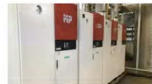
Introduction of High Efficiency Once Through Boiler to Garment Factory, Osaka Gas Co., Ltd., Thailand
