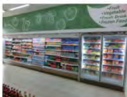
Energy saving at convenience stores, Panasonic, Indonesia
