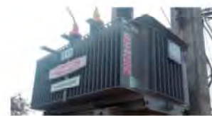
Introduction of Amorphous High Efficiency Transformers in Power Grid, Yuko Keiso Co., Ltd., ①Vietnam, ②Lao PDR
