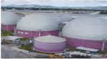
Biogas Power Generation, ITOCHU Corporation, Philippines
