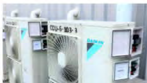
Air-conditioning control system
