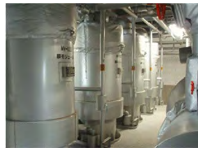
Module of Membranes (Modules install in series)
