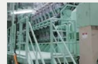
Gas Co-generation System and Absorption Chiller, Kansai Electric Power [Thailand]
