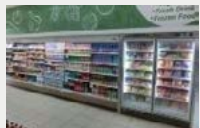
Energy saving at convenience stores, Panasonic [Indonesia]
