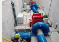
Hydro Power Plant, Toyo Energy Farm Co., Ltd., [Indonesia]
