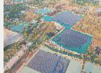
Floating Solar PV, TSB Co., Ltd. [Thailand]
