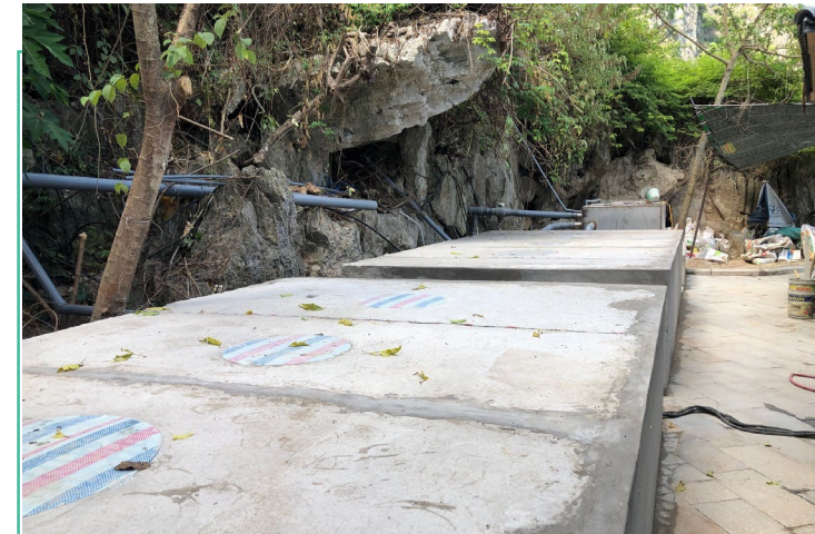
Jokaso installed on Dau Go Island
