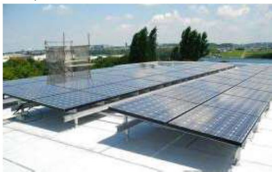
Installation in elementary school
