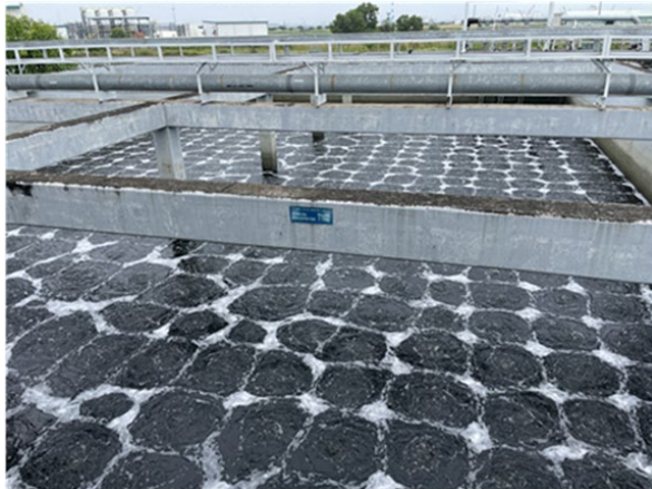
PM3SIP: wastewater treatment facilities
