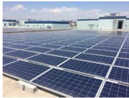
Installation at a sewage treatment plant
