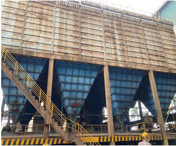
Existing fabric filters
