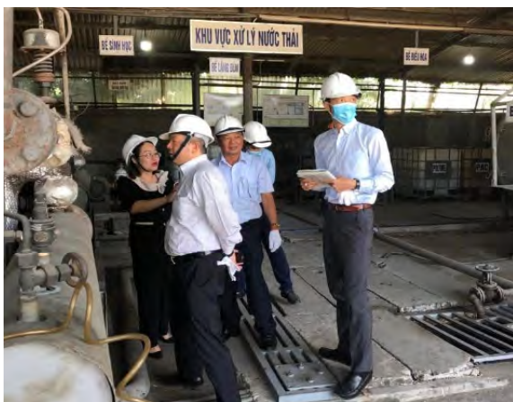
Oil-water separation and wastewater treatment facilities
