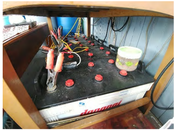
Lead-acid batteries for storing electricity generated with solar PV panels (water raft at location #1).
