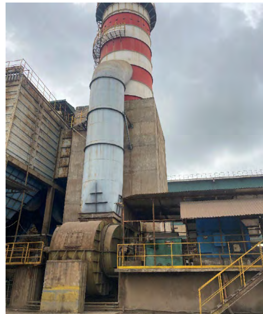
Equipment covered by this survey (side view)
