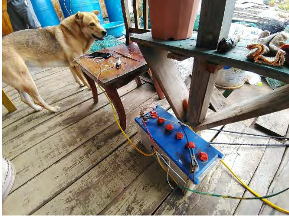
Lead-acid batteries to store electricity generated by solar PV panels (water raft at location #2)
