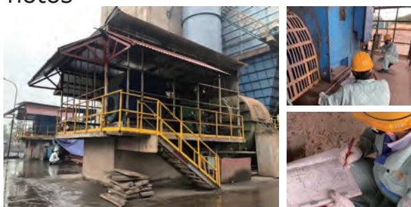
A large industrial blower that is scheduled to be applied for the JCM Model Project and a site survey
