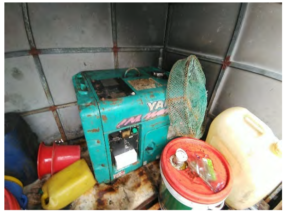
Generator (water raft at location #1)
