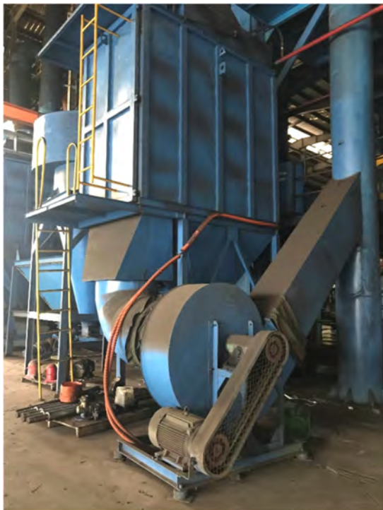
Blowers at the new plant
