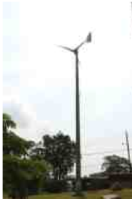
Wind-power generation equipment
