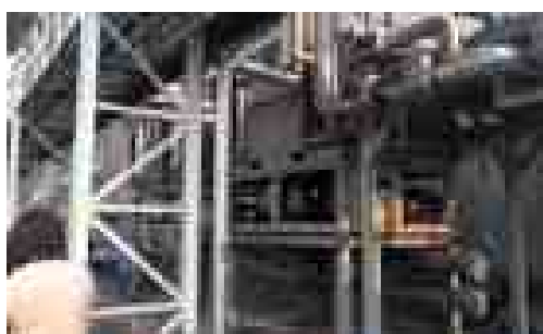
Chiller at the factory
