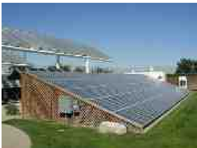
Solar power generation equipment
