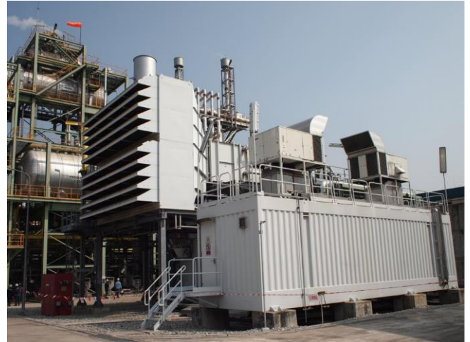
Photo 4. Gas turbine body
