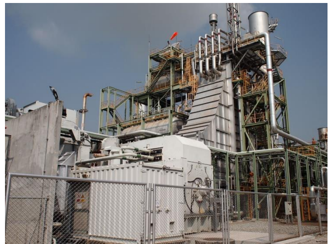
Photo 2. Waste gas boiler
