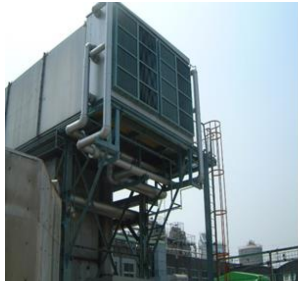
Fig. 3.7 An inlet chiller attached to a gas turbine inlet
