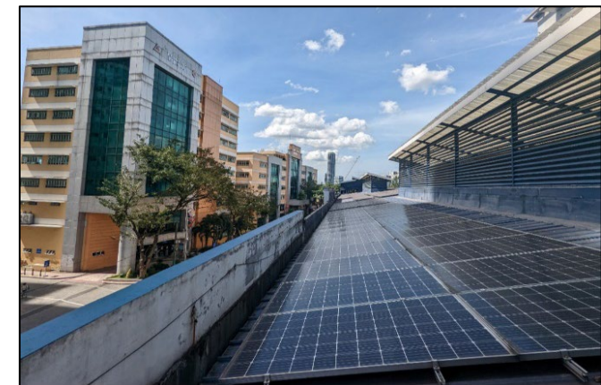
Rooftop solar at Quezon City Hall
