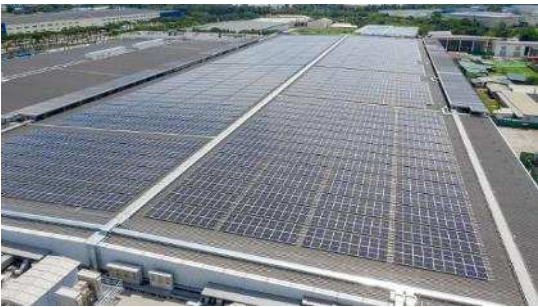
Figure 3-10 Roof-mounted solar panels
