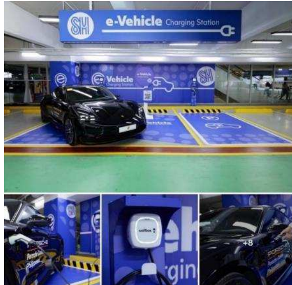
Figure 4-11 E-Vehicle Charging Station
