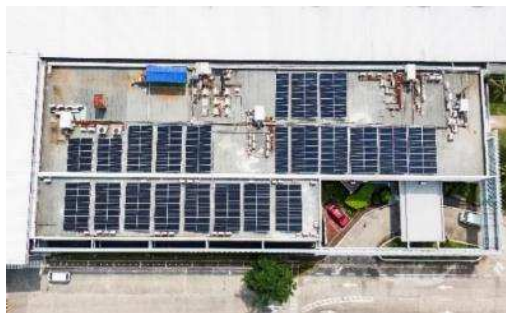
Figure 3-7 Additional solar power generation facilities for factory self-use
