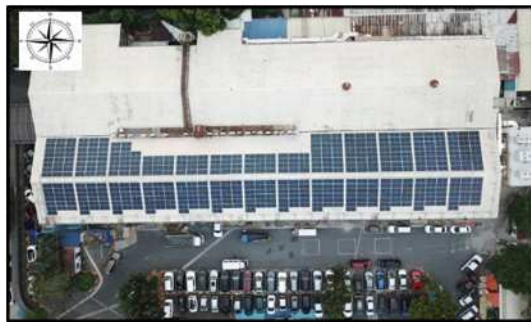
Figure 3-5 Rooftop solar panels at EEI headquarters
