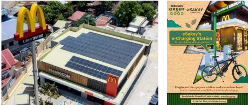
Figure 4-15 Rooftop Power Generation Facility (left) at McDonald's in Quezon City and an Official Poster (right)
