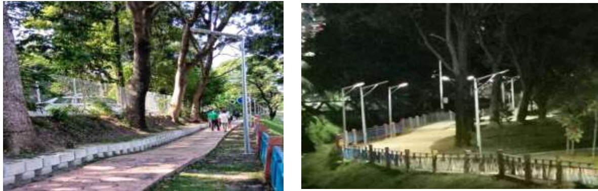
Figure 5.4.2 Solar-powered LED street lights (left) (right)
