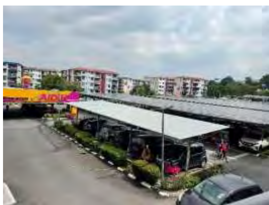
Solar PV at Aeon's Alpha Angle (Aug 9)
