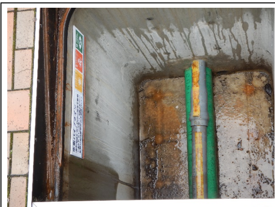
Hydrogen transportation pipe
