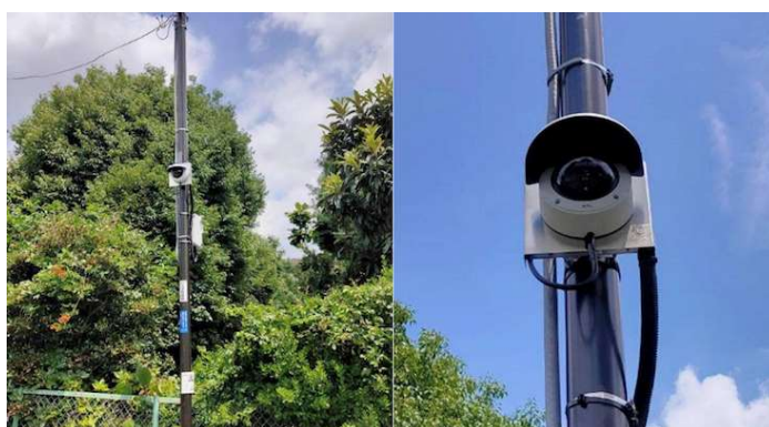
Figure 4-8 IoT streetlight system installed in Suginami Ward
