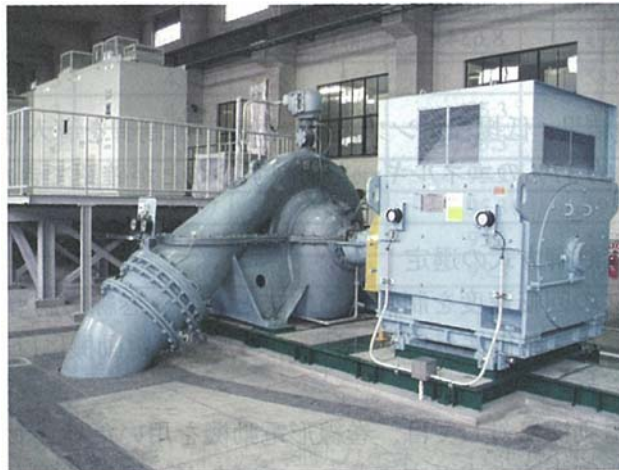
Figure. Example of water pump and inverter
