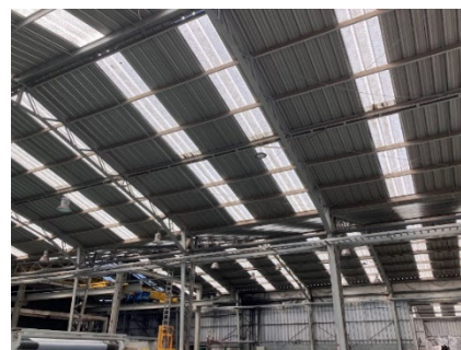
Planned installation location of 2.0MW solar PV system (Roof of plastic factory in Renca)
