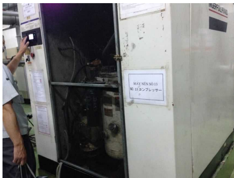
Photo 3.1.5 Checking the operation status of the compressor
