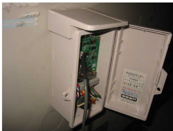
Photo 3.1.3 Be One control equipment
