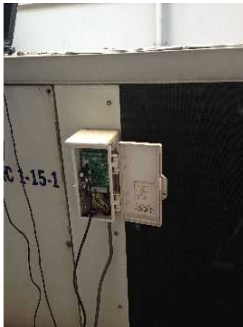
Photo 3.1.4 Be One on the outside unit of air conditioner
