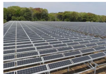
Photovoltaic power system
