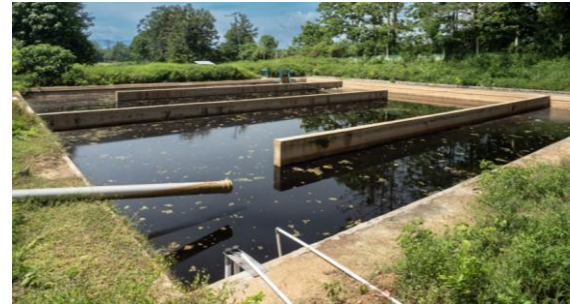
Existing leachate treatment plant
