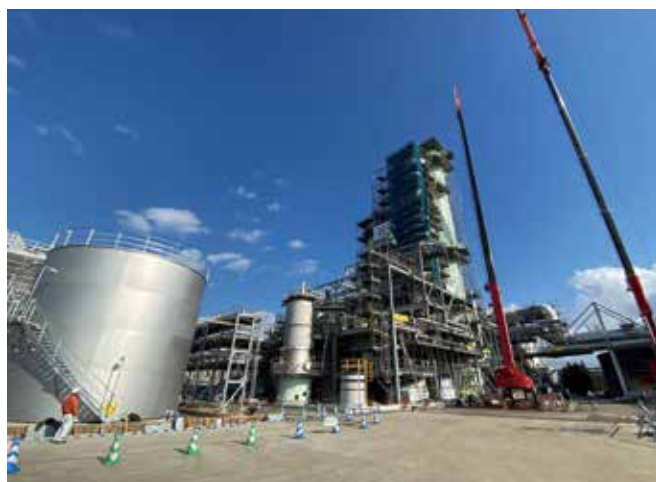
CO 2 capture demonstration facility under construction (as of the end of January 2020)
