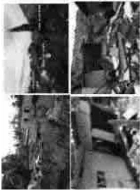
Ground movement and damages to houses due to deepening of the drainage canal; which removed toe support in the toe region at the South-West section in Oct 2012
