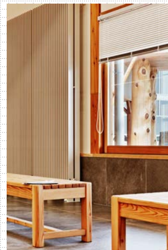
▲ Air-conditioning system using geothermal heat (Radiant panels)
