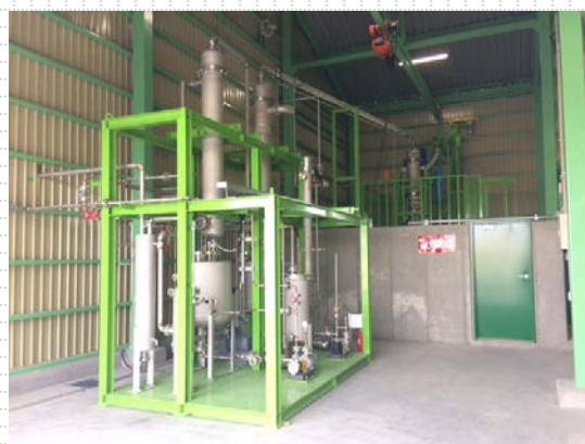
▲Oil conversion equipment
