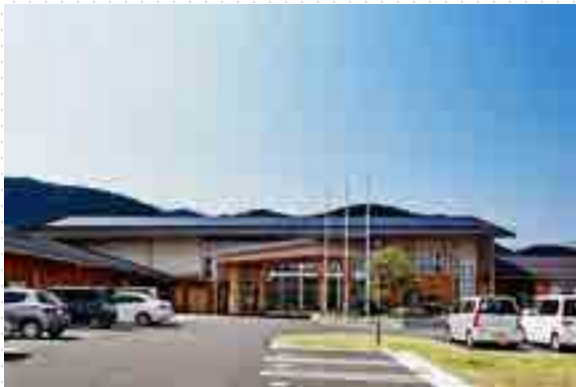
▲ Photovoltaic power generation system for the village hall building
