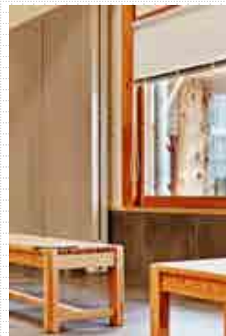
▲ Air-conditioning system using geothermal heat (Radiant panels)
