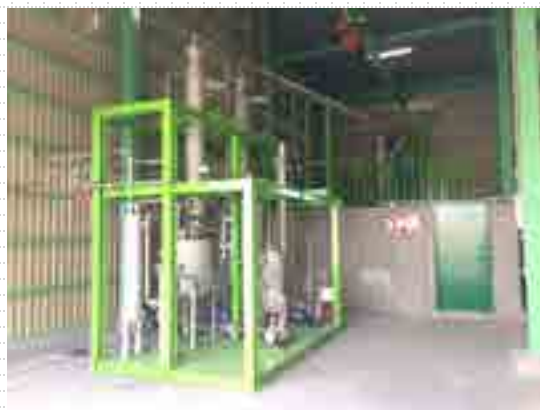
▲Oil conversion equipment
