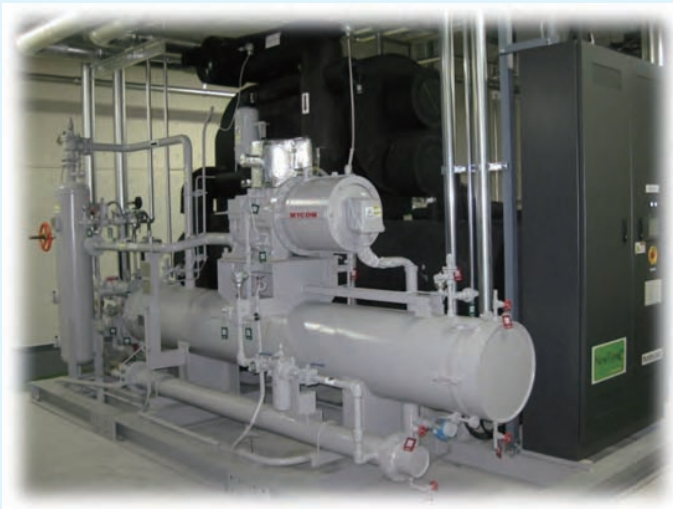
NH3/CO2 refrigeration system (+05°C)
