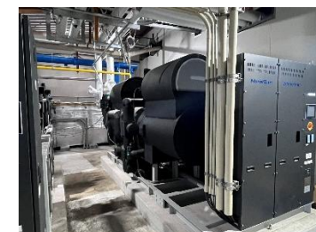
NH 3 ／CO 2 冷媒冷凍機本体②
