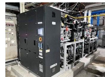
NH 3 ／CO 2 冷媒冷凍機本体①
