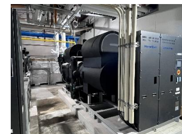
NH 3 ／CO 2 冷媒冷凍機本体②
