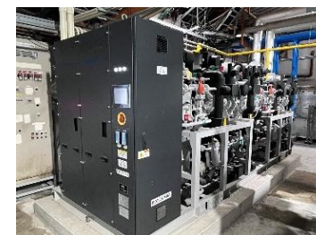
NH 3 ／CO 2 冷媒冷凍機本体①
