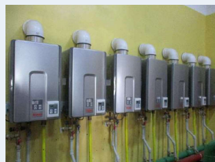
Gas water heaters
