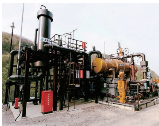
Binary geothermal power plant
