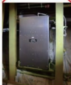
CME Continuous CO 2 Measuring Equipment
