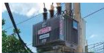
Amorphous transformers in power distribution, Yuko-Keiso, Vietnam
