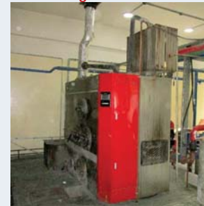
Existing coal-fired HOB
