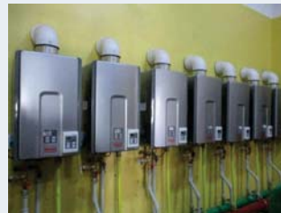
Gas water heaters
